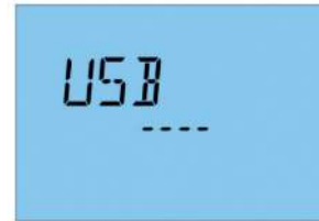
Fig. 65: Checking the USB power supply unit
